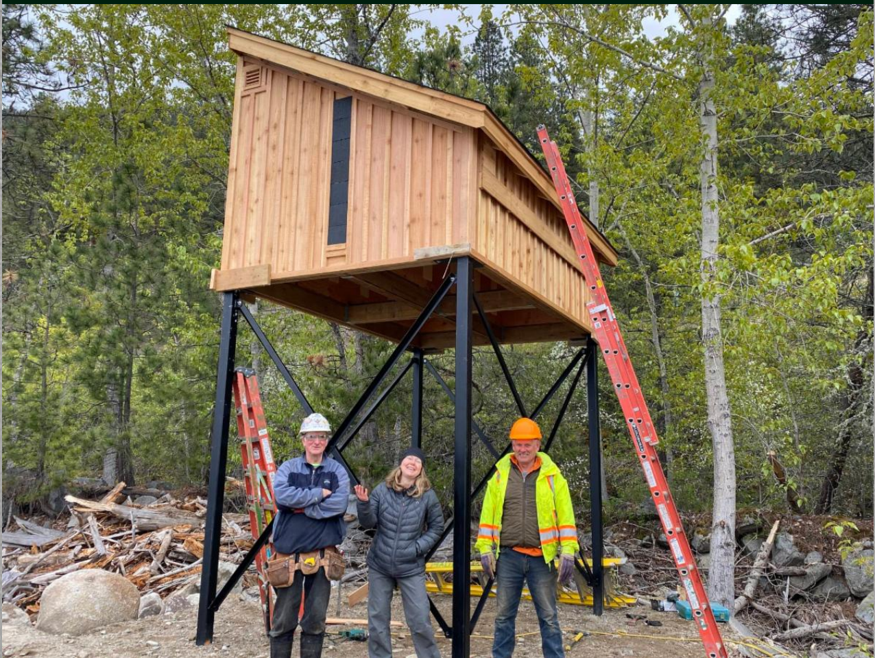
The new Kuskanook Bat Chalet. From left: Derick Todd (Malibu Construction), Dr. Cori Lausen (Wildlife Conservation Society Canada), Geromy Piva (Piva Mechanical Industrial Crane Services). Photo: WCS Canada
